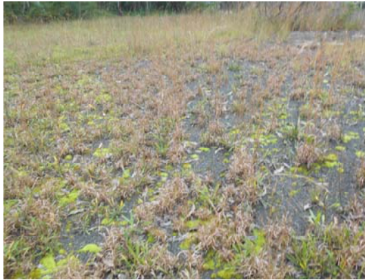
Photograph 25: View of bitumen gravel on surface at the southern portion of 14-16 Orion Road (June 2015)
