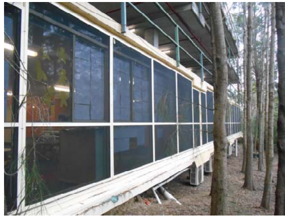
Photograph 14: North-western end of the carpark showing air conditioning units underneath the Childcare Centre, 18-20 Orion Road (June 2015)
