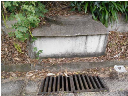
Photograph 19: View of stormwater/drain system structures observed at the vicinity of the Childcare Centre, 18-20 Orion Road (June 2015)
