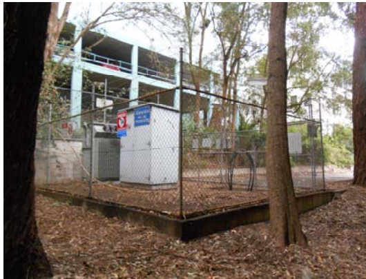
Photograph 17: Electric Substation located on the south-western portion of 18-20 Orion Road (June 2015)
