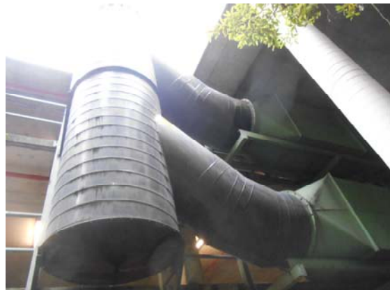
Photograph 16: View of the end pipe part of the carpark exhaust pipe system, on 18-20 Orion Road (June 2015)
