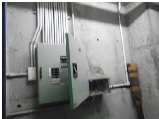
Photograph 10: Building unit room located in carpark area underneath the building footprint on 18-20 Orion Road (June 2015)
